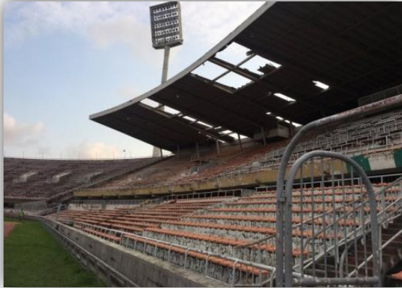
Falling Off Roof of Part of the Main Bowl
